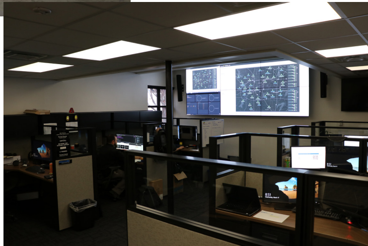
Completed construction on the Network Operations Center at Tarrant County 9-1-1 District (2020)
